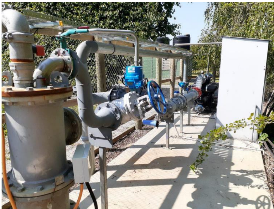
Figure 1: Photo of a MAR trial injection well (source: van Nieuwker and Cudmore 2021) 6
