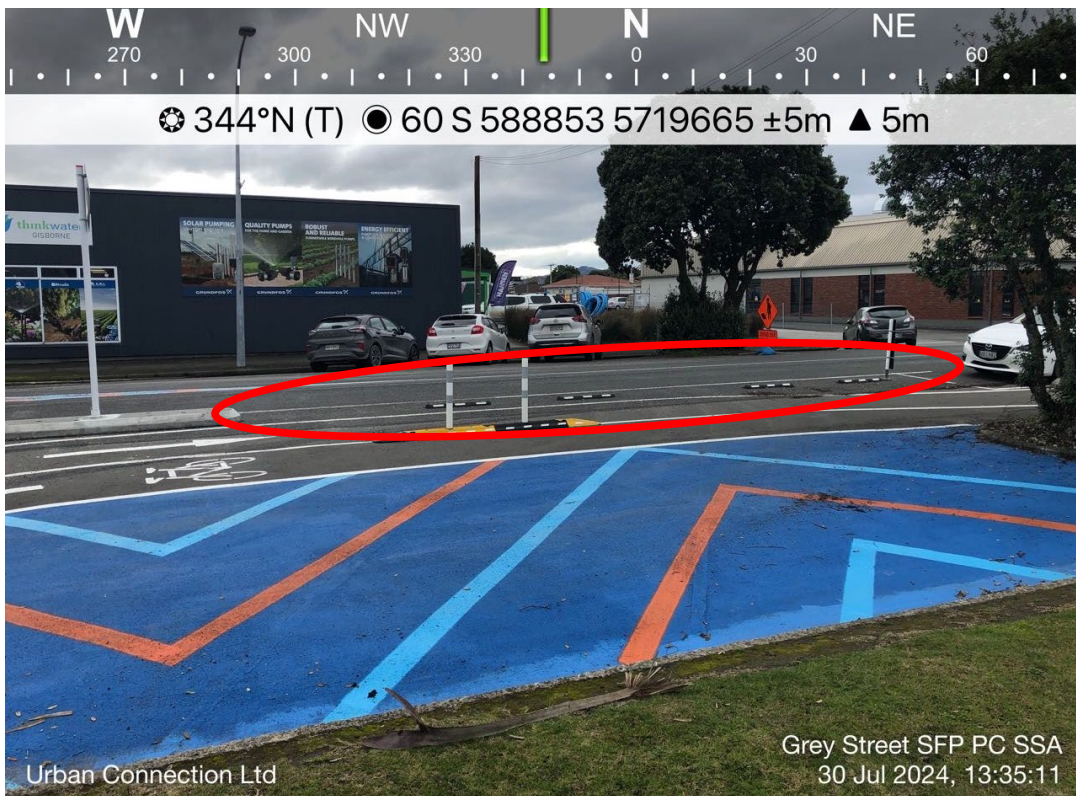
Figure 4.4-5 – Section with no physical deterrent (concrete kerb separators) on the north side of the Grey Street/Kahutia Street intersection
