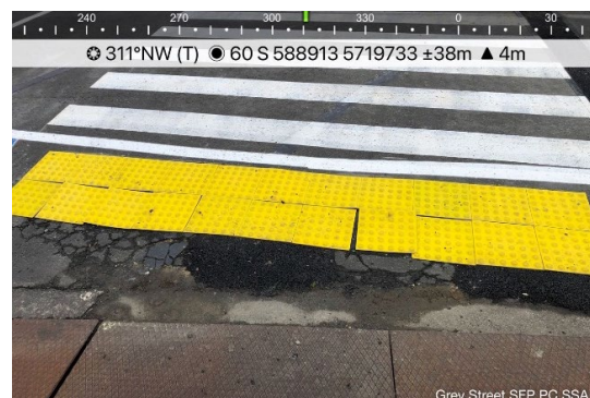
Figure 4.4-18 – No directional tactile indicators and poor installation of warning tactiles at the pedestrian crossing on Grey Street
