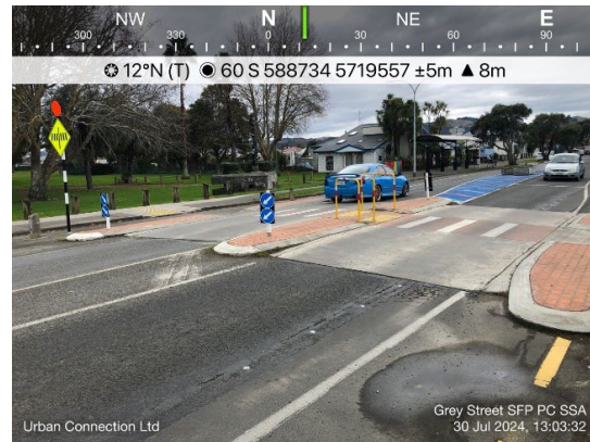
Figure 4.4-32 – Missing white triangles at raised pedestrian crossing
