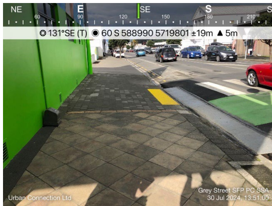
Figure 4.4-21 – No directional tactile indicators at the pedestrian crossing on Childers Road
