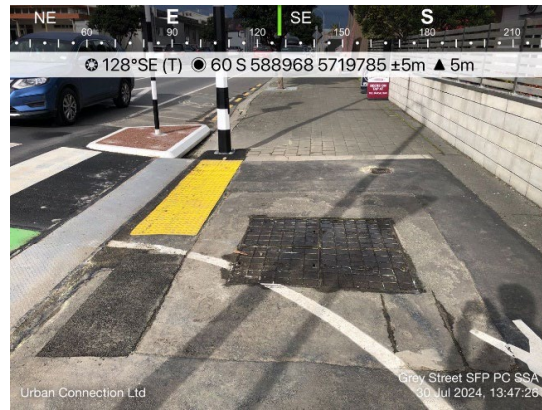
Figure 4.4-20 – No directional tactile indicators at the pedestrian crossing on Childers Road
