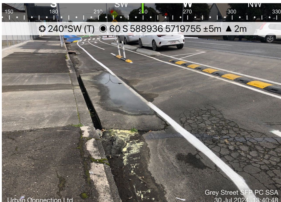
Figure 4.4-27 – Ponding adjacent to the cycle lane
