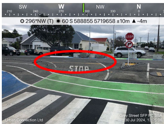
Figure 4.4-29 – Faded limit line at the Grey Street/Kahutia Street intersection
