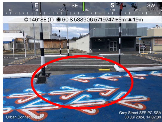
Figure 4.4-22 – No warning and directional tactiles at the pedestrian crossing on Grey Street
