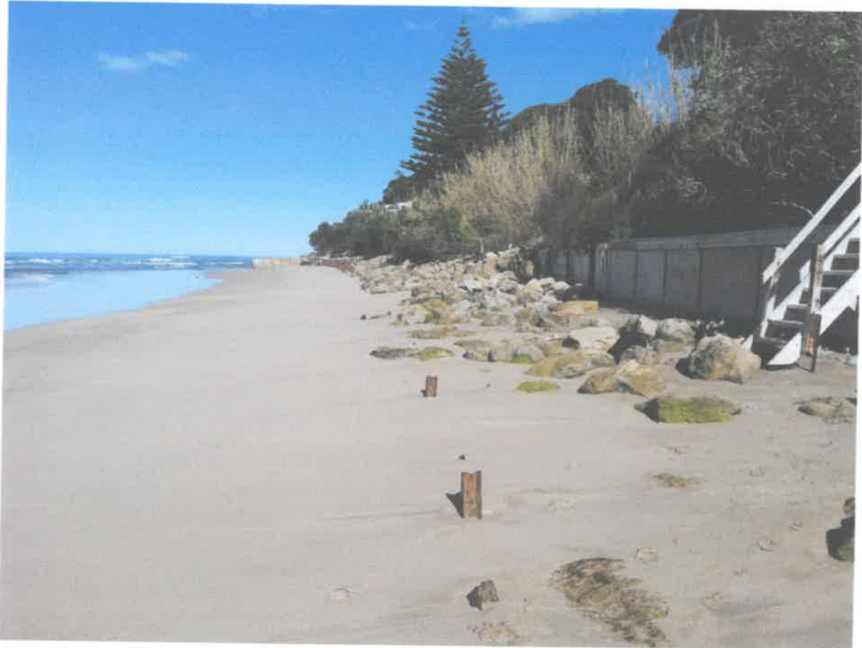
Photograph 2: Sea frontage 60 Murphy Rd, 7.8.2017 showing the rail irons emerging when the sand level is low.
